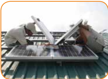
PV installation (Source: ECC 2013)
