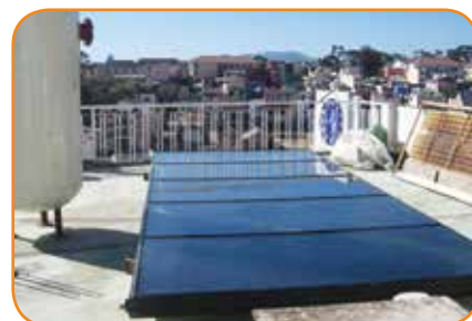
Installing a hot water system using solar power in Dalat City project (Source: www.enerteam.org)
