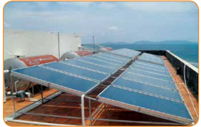
Solar water heater of a town house (Source: BK-IDSE Co 2012)
