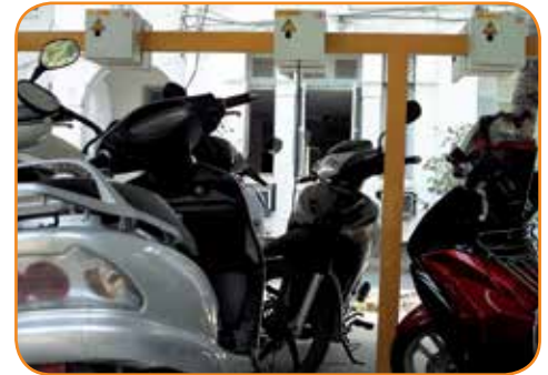
Docking station for electric bikes at ECC-HCMC (Source: Michael Waibel 2013)
