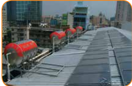
Solar water heater system Majestic Hotel, HCMC (Source: en.bk-idse.com)
