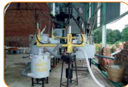
Project about brick kiln combined with a rice husk gasification system (Source: ENERTEAM)
