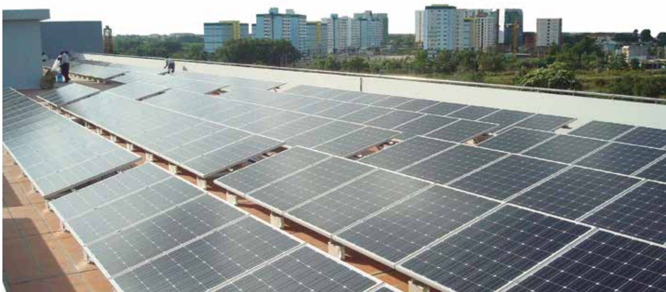
The 50.16 KWp On-Grid and Back up combined system at the Institute for Environment and Resource - IER HCMC (Source: Redsun 2013)
