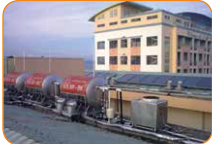
Solar water heater system Cap Saint Jacques Hotel - Vung Tau (Source: en.bk-idse.com)
