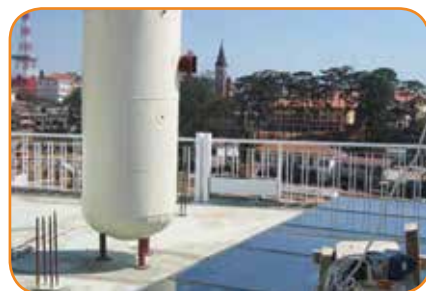
Installing a hot water system using solar power in Dalat City project (Source: www.enerteam.org)
